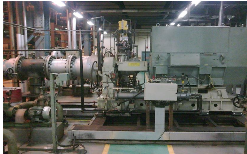
600 kW St. condensing GMR, Diesel PP Basin Bridge, Chennai
