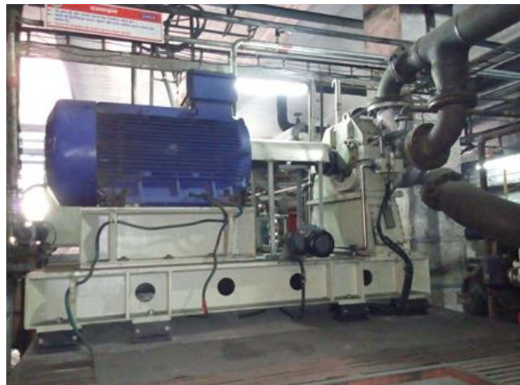
360KW Turbine at Durga Textile
