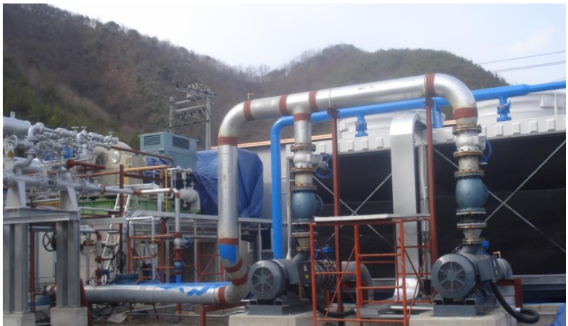
640 kW Turbiner at Chemical Plant
