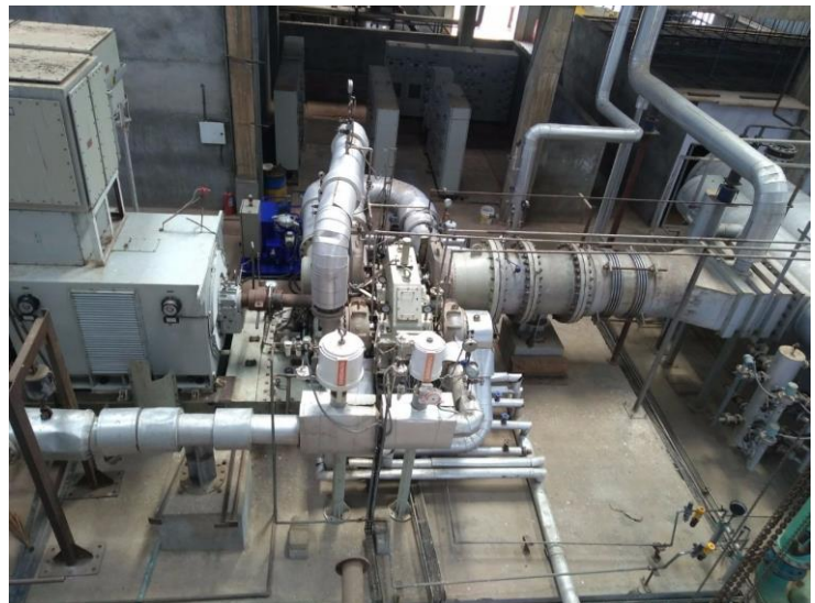
3 MW condensing Turbine at Harihar
