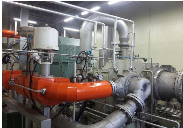
South Korea 3MW waste incineration
